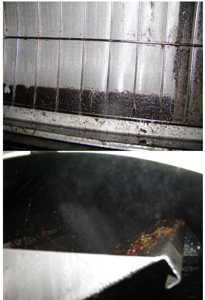
Figure 3: Solids trapped by the screen, displaying the water level, left behind after being drained (top) and the spray bar removing solids from the screen (bottom) (HMGA Water Project)
