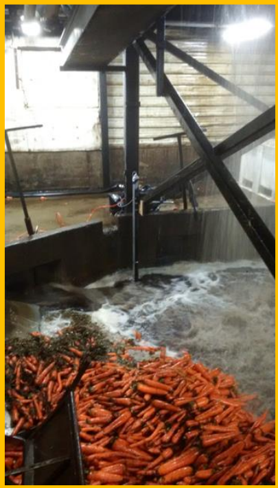
Sensor installed in Dump Tank
