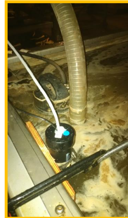
Sensor installed in Polisher Tank
