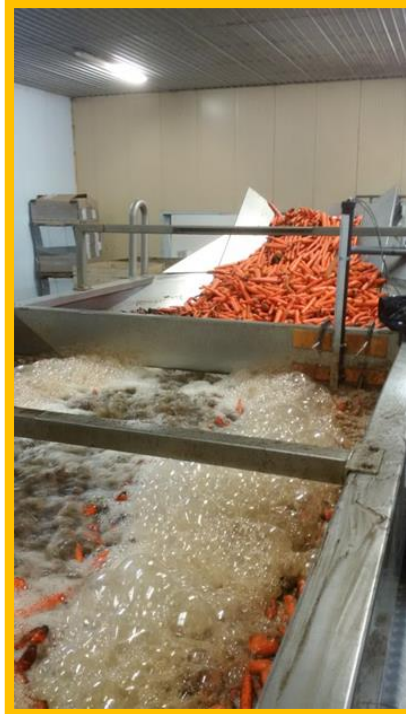
Sensor installed in Dump Tank
